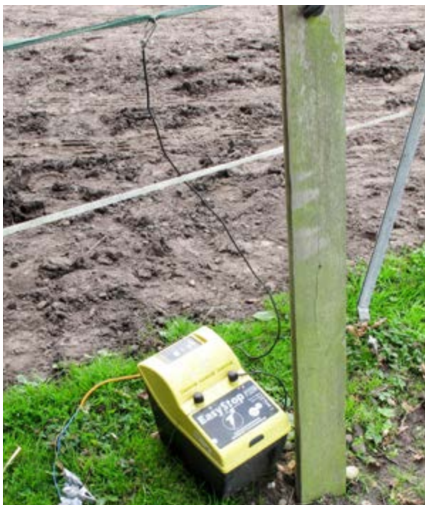
ELECTRIC FENCE POWER UNIT (NB BATTERY NOT CONNECTED)
