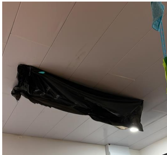
Figure 12: Dale's leaking ceiling.
