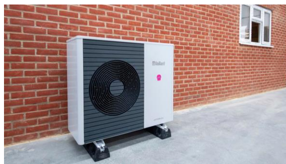
ASHP on anti-vibration mounts but near opening
