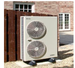
Air Source Heat Pump (ASHP)
